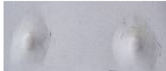
<Failure of Rivet>
